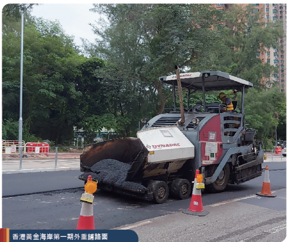
香港黃金海岸第一期外重鋪路面 Road resurfacing works outside Hong Kong Gold Coast Phase I
