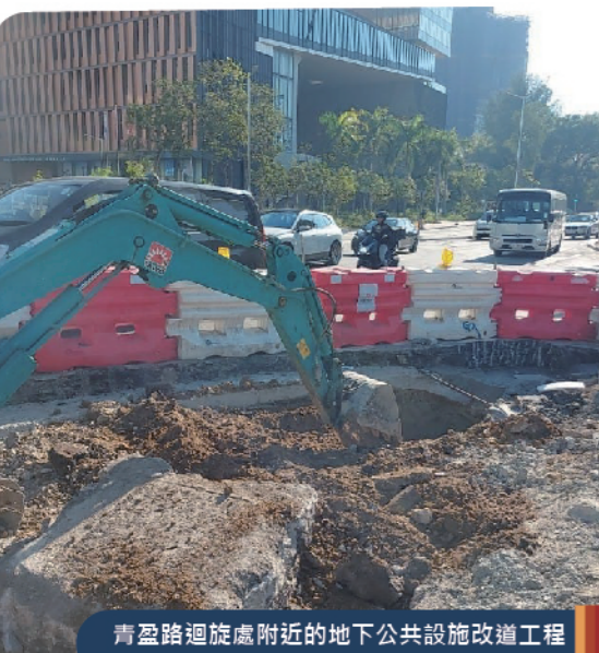
青盈路迴旋處附近的地下公共設施改道工程 Underground utility diversion works near Tsing Ying Road roundabout
