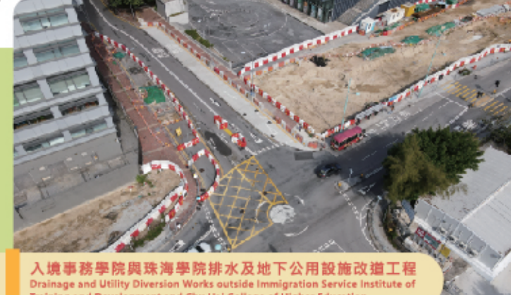
幹華小築外圍隔音屏土地勘測工程 Ground Investigation Work for Noise Barrier outside Villa Cornwall
