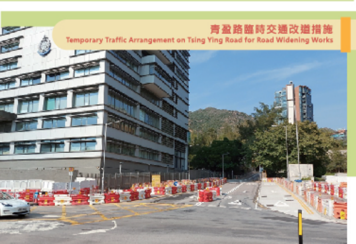
入境事務學院與珠海學院排水及地下公用設施改道工程 Drainage and Utility Diversion Works outside Immigration Service Institute of Training and Development and Chu Hai College of Higher Education
