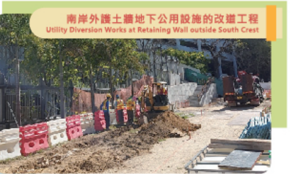
麒麟崗公園升降機排水系統工程 Construction of Drainage System for Lift at Ki Lun Kong Public Park
