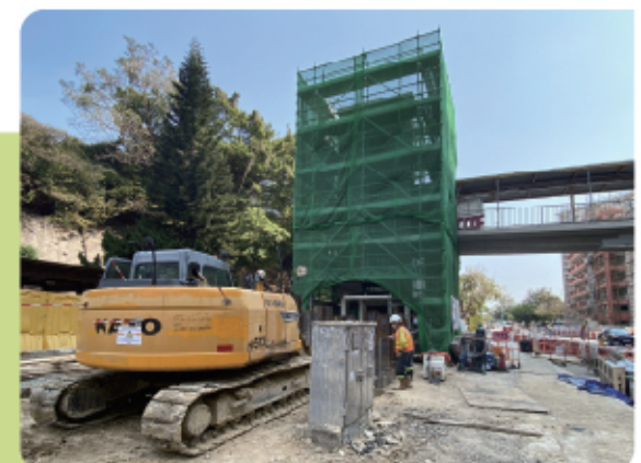
滿發里旁護土牆工程 Construction of Temporary Support for Retaining Wall near Mun Fat Lane
