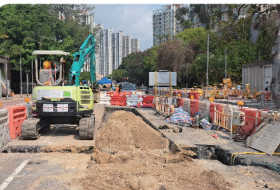
青霞里附近建造中央分隔帶及進行排水渠工程 Construction of central dividing strip and drainage works near Tsing Ha Lane
