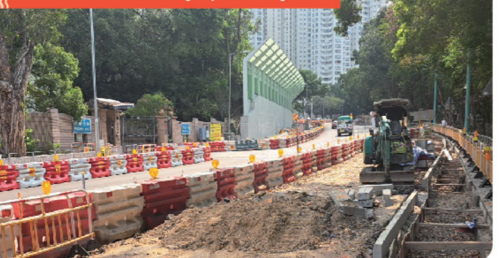
青碧街附近的道路工程及交通訊號系統安裝工程 Road works and installation of traffic signal system near Tsing Bik Street
